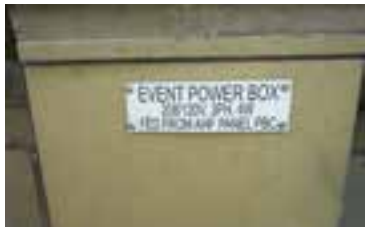
Labeling for Event Power Box
