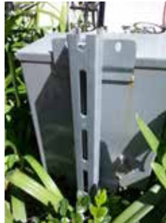
Enclosure on Unistrut in Planter
