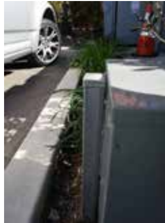
Enclosure on Unistrut
