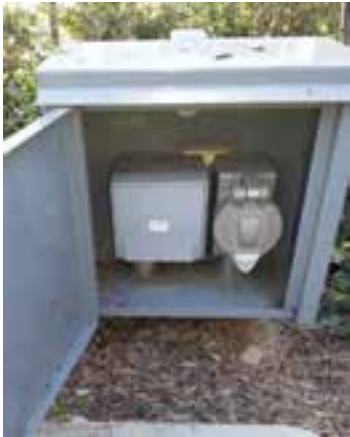
Lockable Enclosure with Outlets
